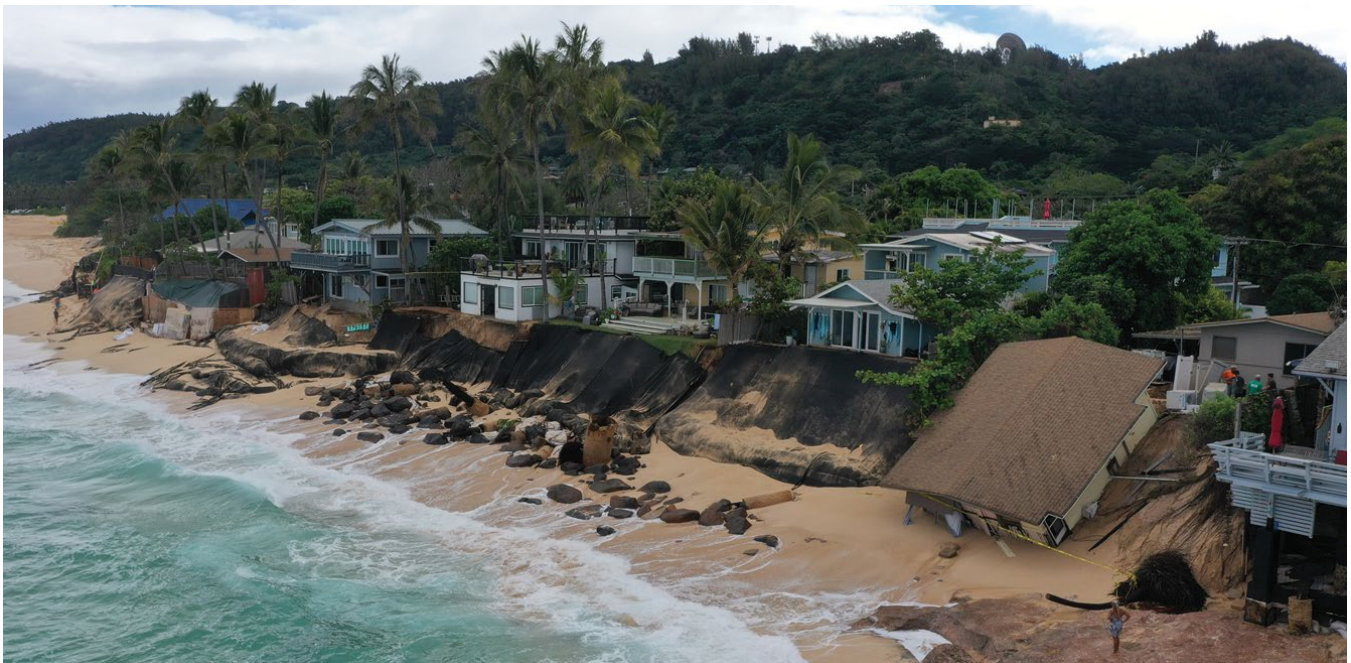
Collapsed home, tarps, and other temporary erosion control measures impair beach access between Rocky Point and Sunset Beach Park, North Shore, O'ahu. (© Shellie Habel, Sea Grant / DLNR)
